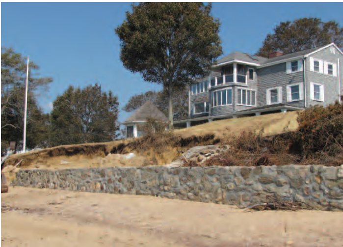
Erosion behind a seawall in Madison due to Tropical Storm Irene
