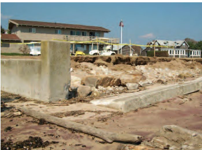
Tropical Storm Irene caused erosion and seawall damage in Fenwick/Old Saybrook.
